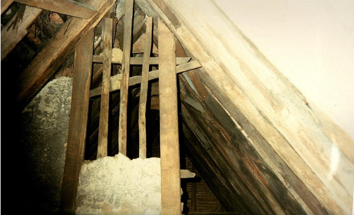
Number 1264. Roof space partition from east. Wattle and daub. Rafters straight butt purlin.
