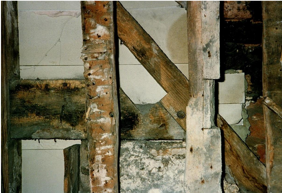
Number 1268. November 1991. Purlin has been removed during later renovation
