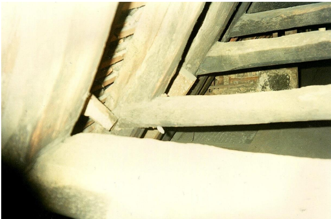
Number 1264. October 1989. Roof inside. Sole plate, rafters, detail of joint to beam.
