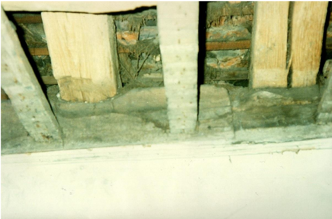
Number 1264. October 1989. Bedroom. Purlin & rafter showing joint shaped with axe or adze.
