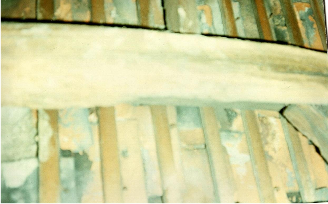
Number 1264. October 1989. Rafters, roof tiles on battens, probably Victorian. Carpenters marks obscured by flash.
